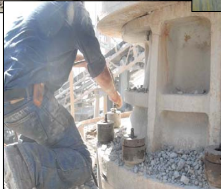
Top Shell retained by HydraNuts
